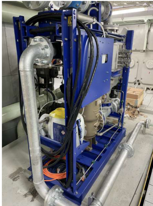
Complete installation of Ballast Water Treatment Systems
