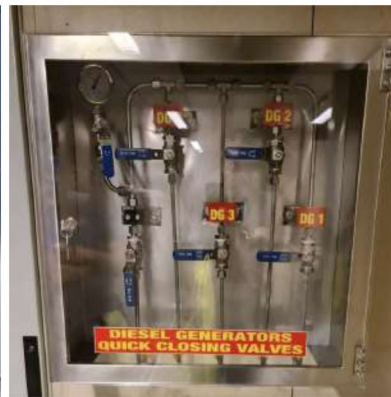
Complete Fuel Flow meters / quick closing valves installation (including compressed air plant and electrical wiring)
